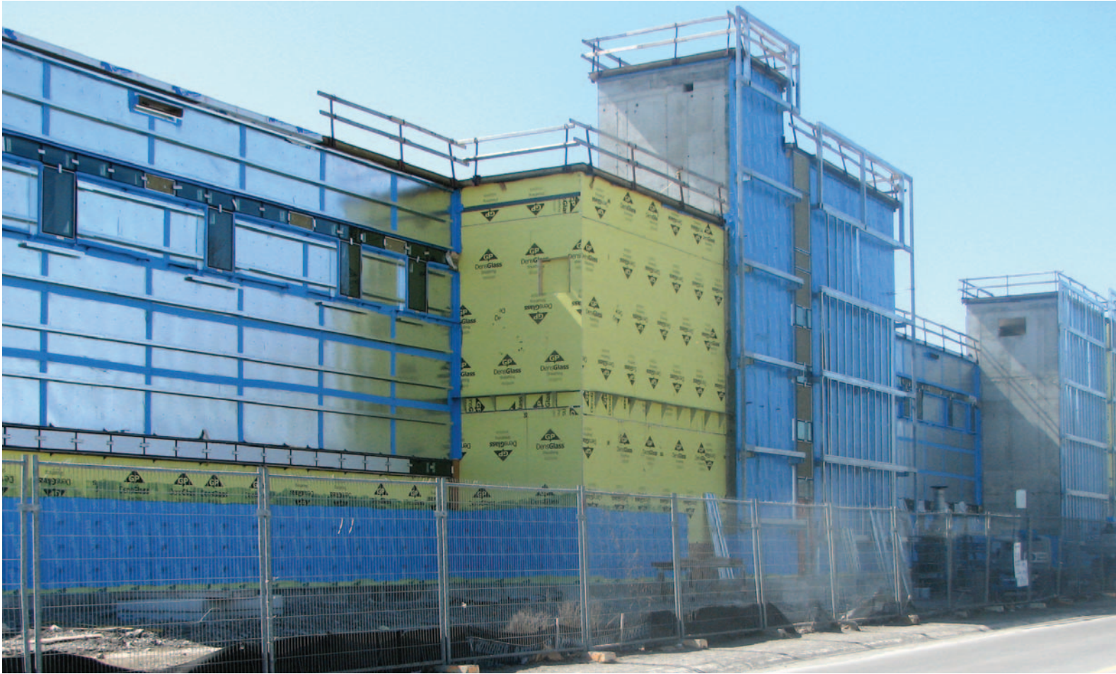
New TDL Distribution Centre on Innovation Drive, Kingston
